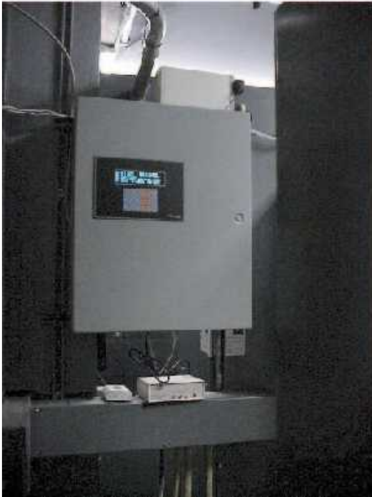
Figure 5 – The power monitoring System in the electrical room at Allied Converters
