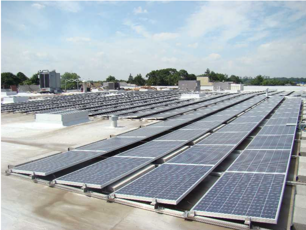
Figure 12 – 50 KW roof mounted solar array
