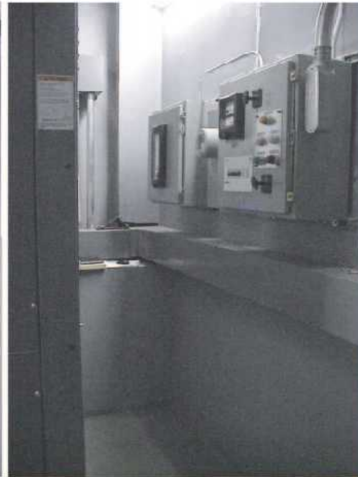
Figure 9 – Protective relays for the CHP system
