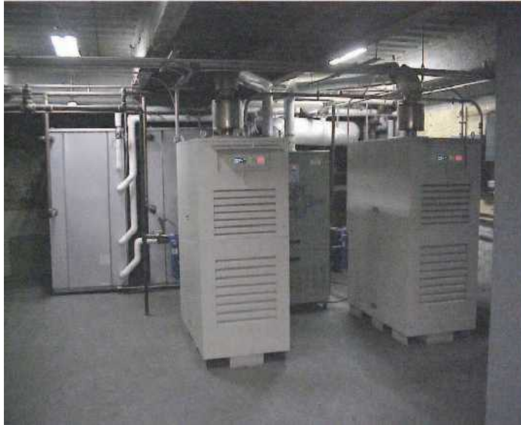
Figure 7 – CHP System Micro turbines are in the foreground. The heat exchanger is the cabinet to the rear and center of the two micro-turbines. The two tall, gray cabinets to the rear left are 10 ton absorption chillers that use the hot water from the heat exchanger to generate 43 degree chilled water during the cooling season.
