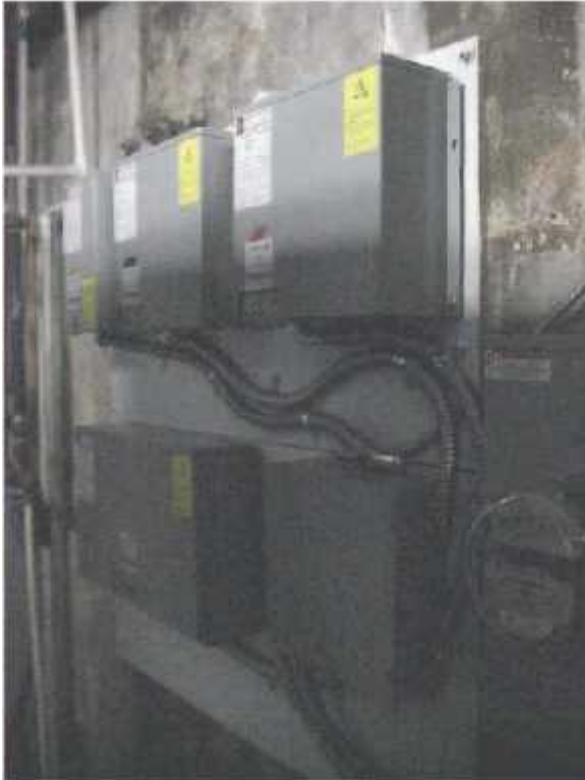
Figure 10 – 45 KVAR power factor correction at the utility service entrance. These devices are connected to and disconnected from the service by the monitor shown in Figure 5. The solar power meter is in the foreground on the far right
