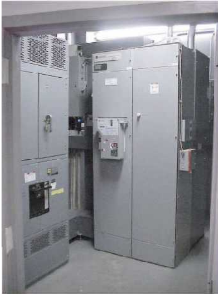
Figure 8 – Main Utility Circuit Breaker (left) and 1600 Ampere transfer switch (right). Automatically disconnects the internal service from the utility during a power failure.
